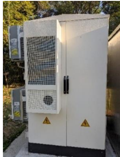
Fig. 2 - Photo of Ground-Mounted BESS Deployed in LV Network
