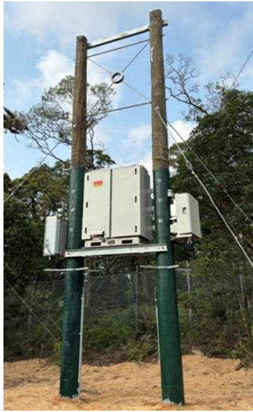
Fig. 5 - Photo of P-BESS Trial Installation
