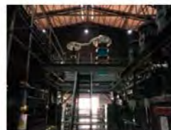
Generation Substation by CHAN Wan Yu
