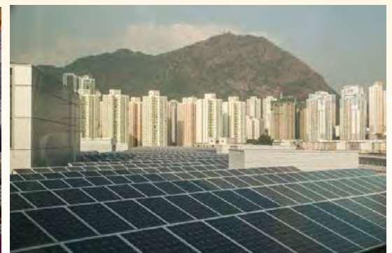
Sea of Photovoltaic Panel
