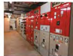
The Second Essential: Main Switchboard by CHEUNG Hon Lun
