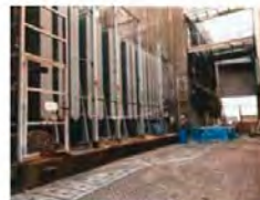
The First Essential: Transformer
