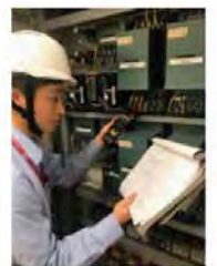
Protection Relay Testing
