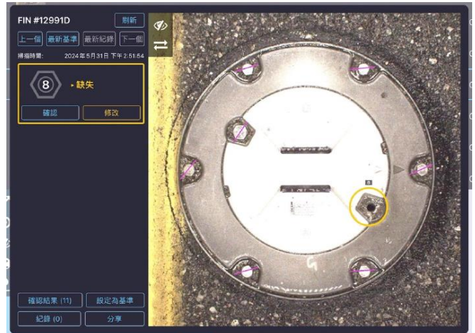
Fig. 1 - The Missing Bolt was highlighted in the Operator Mobile Device
