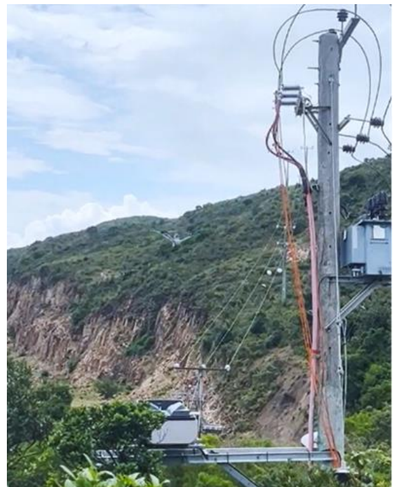
Fig. 1 - A Drone Docking System installed in a 11kV Distribution Pole at Sai Wan
