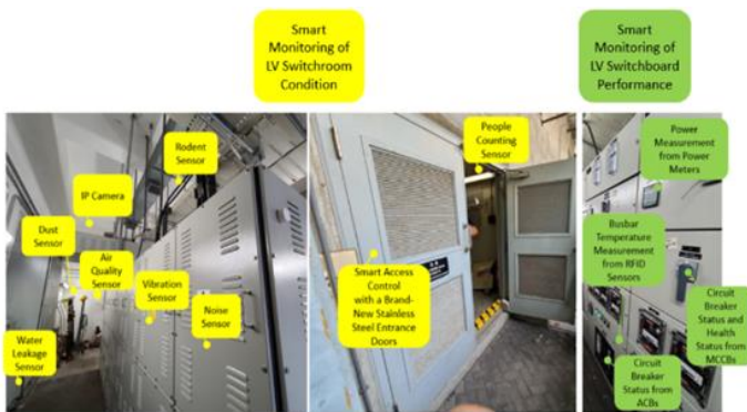
Fig. 16 - Key Components of Smart Switchroom Monitoring
