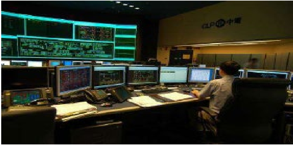
Power System Control Centre
