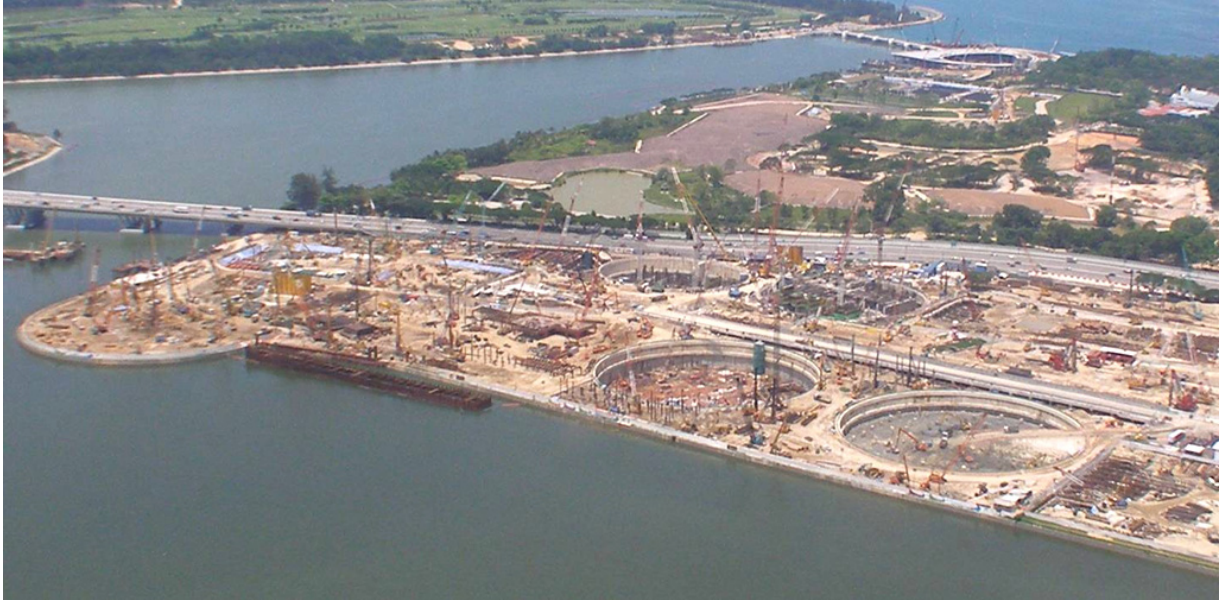
Plate 6: View of the Marina Bay Sands Integrated Resort taken from the south west showing the two 120m diameter circular excavations in the lower foreground, the Hotel Peanut in the upper centre and the 130m diameter outline on the left hand side
