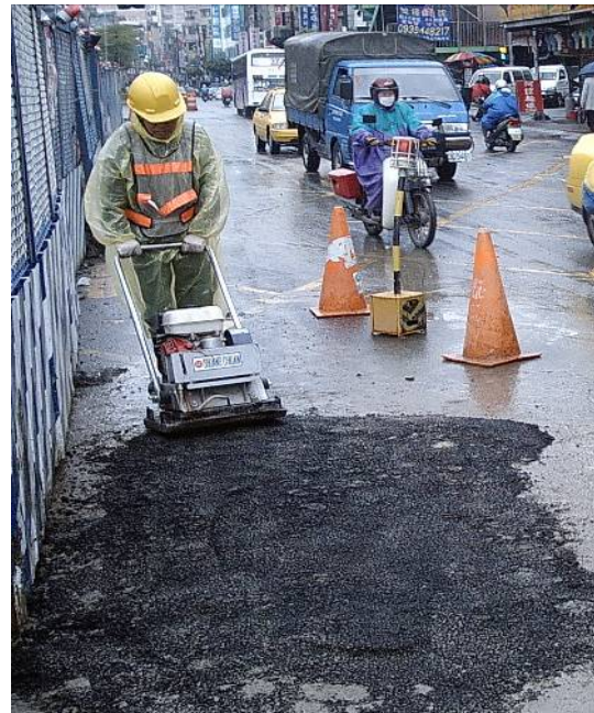
Trench collapse, causing adjacent ground settlement. Guide wall movement, construction shall be stopped.
