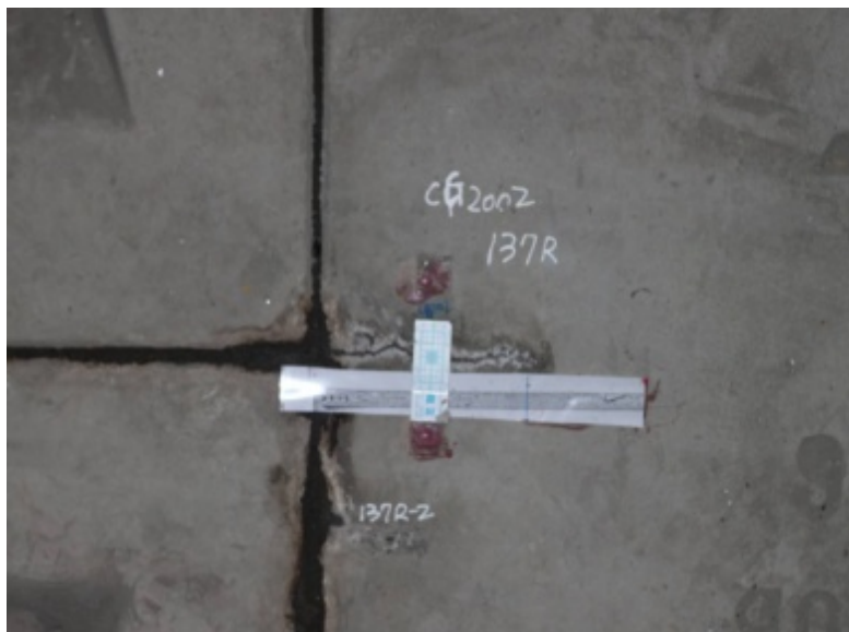
Plate 2: Cracks on linings
