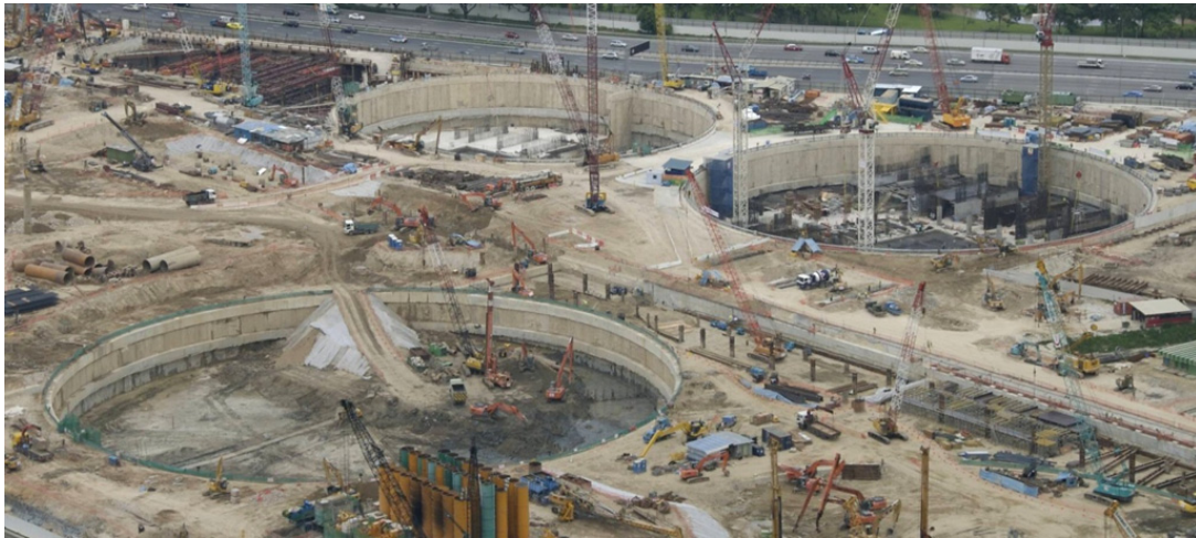
Plate 10: View showing vehicle ramp within the northern 120m diameter circular excavation with Hotel Peanut and 103m circular excavation in the background
