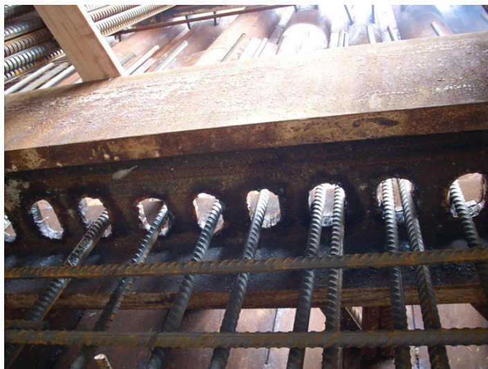
Plate 3: Clash between temporary and permanent works
