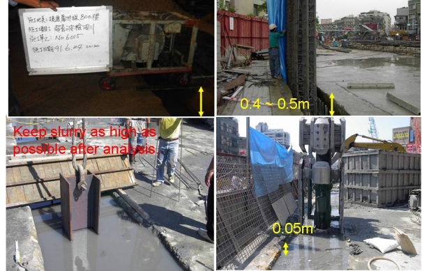
Figure 3-7: Slurry raise from 0.4m to 0.05m below guide wall surface for O47 station.
