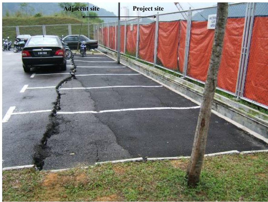
Figure 7: Site conditions of adjacent lot after the incidence of wall and ground distresses (Northward view)
