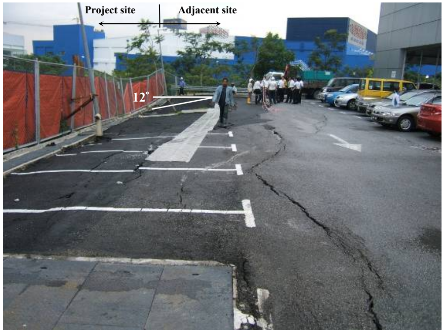
Figure 6: Site conditions of adjacent lot after the incidence of wall movement and ground distresses (Southward view)
