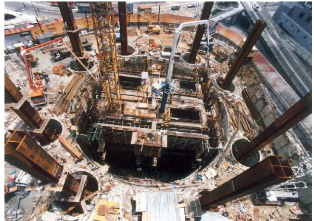
Plate 2: View of the core and mega columns prior to the excavation of the overall basement at the Cheung Kong Centre
