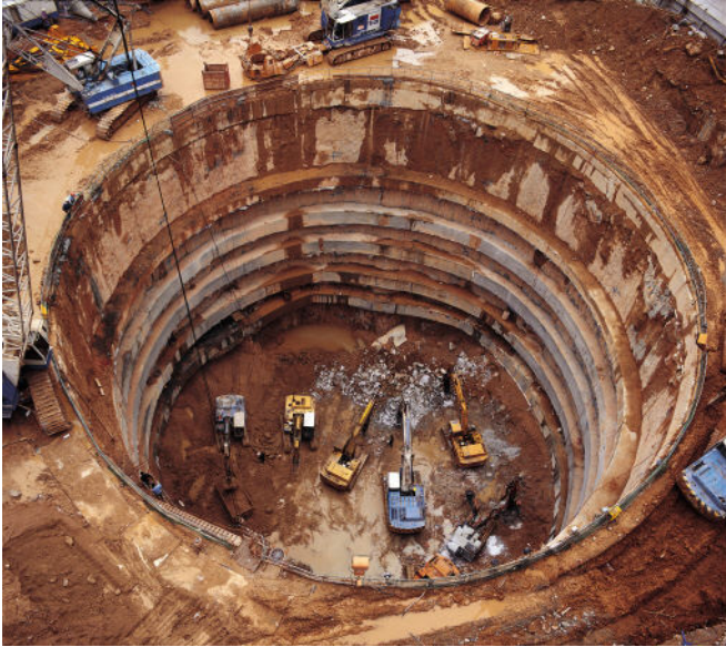
Plate 1: View into the excavation for the core of the Cheung Kong Centre
