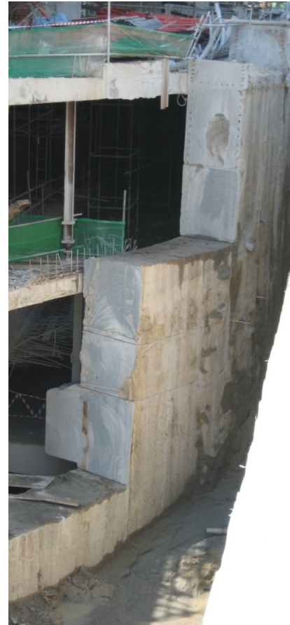
Plate 8: View of the Hotel 103m diameter circular diaphragm wall being removed by wire cutting into blocks
