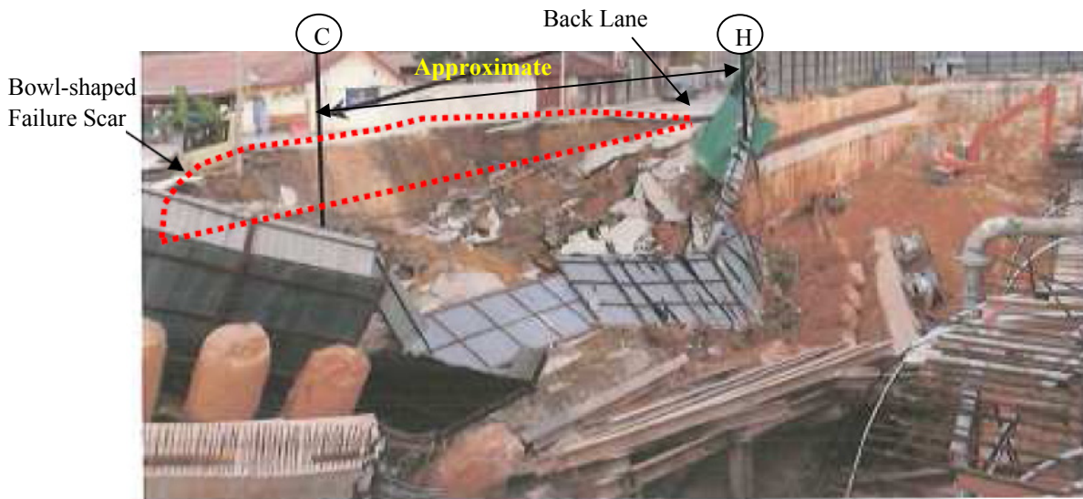
Figure 14: Collapsed CBP between Gridlines C and H
