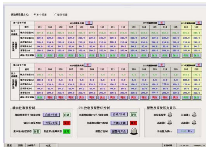
Figure 6: Control and Monitoring Panel for 4th and 5th Layers of Strut
