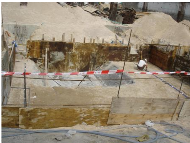
(a) FBG sensing tubes for settlement profile measurements
