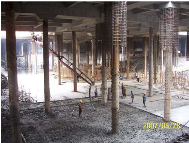
Figure 19: An interior view of the excavation showing steel tubes used as vertical support
