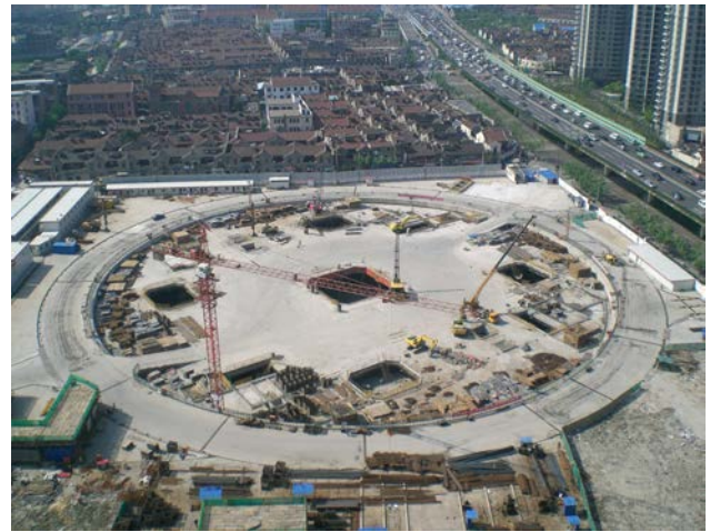
Figure 18: An aerial view of the project showing the completion of the roof slab
