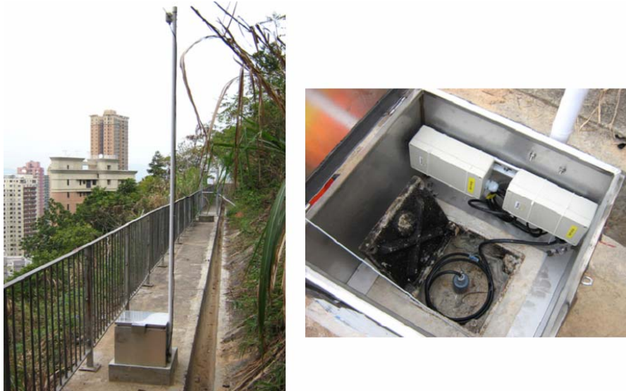
Figure 4: External and internal view of wireless datalogger enclosure at top of borehole
