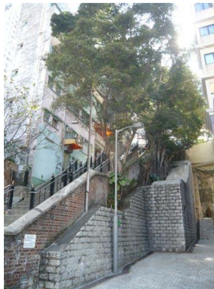
Plate 2: Wall trees were still in good condition after five years of the works (photo taken on 7 February 2011).
