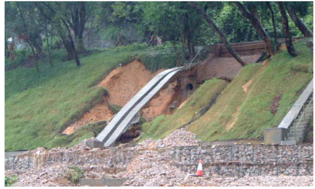
Plate 8: Failure of a compacted rockfill slope at South Lantau Road in 2003
