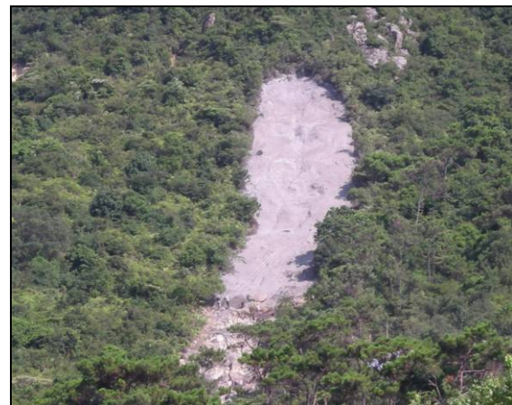
Plate 5: The shotcrete at failure scar of NC6
