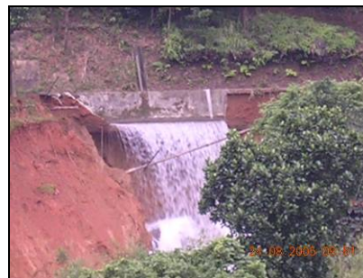
Plate 2: Water scouring out the downslope area
