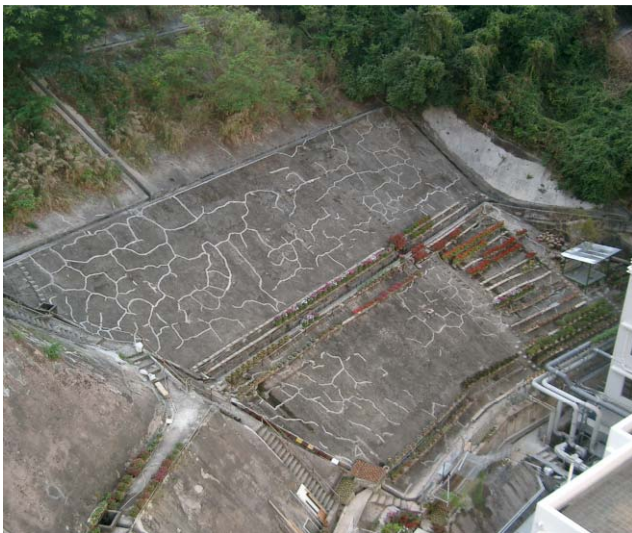
Plate 9: The distressed slope below Stubbs Road reported in 2004
