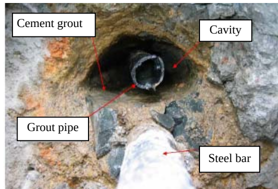
Plate 11: Absence of grout on the upper part of drillhole
