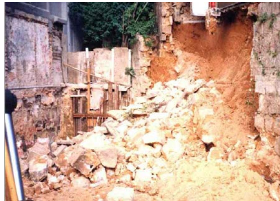
Figure 8: Failure of a Typical Masonry Wall
