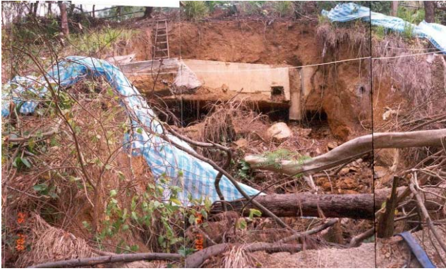
Plate 7: Major failure of a recompacted fill slope at Castle Peak Road in 2000
