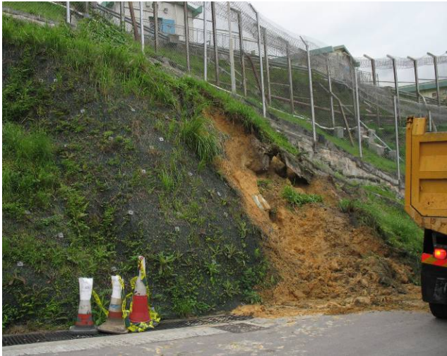
Plate 5: Minor failure (10 m 3 ) at Tai Lam Correctional Institution in 2009
