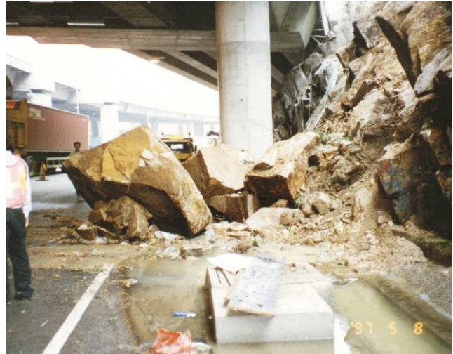
Plate 6: Relatively large detachment (23 m 3 ) at Kwai Chung Road in 1997
