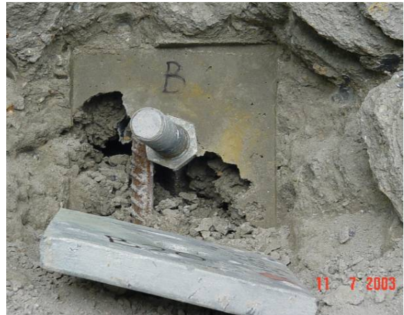
Plate 17: Voids observed below the bearing plate
