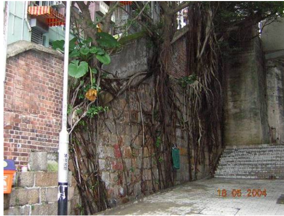
Plate 1: Proposed mass wall was in conflict with the roots of existing wall trees at Feature No. 11NW-A/R88 in Ladder Street (photo taken before works on 18 May 2004).
