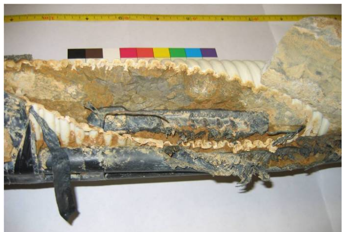
Plate 18: Doubtful grout integrity detected in completed nail
