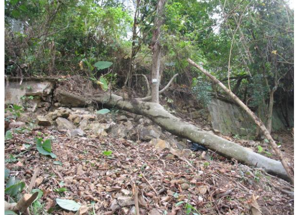
Figure 3: Distressed masonry wall
