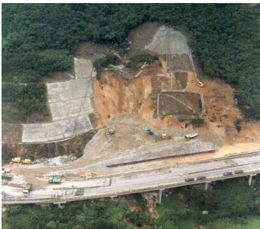
Figure 17: Landslide at Ching Cheung Road in 1997
