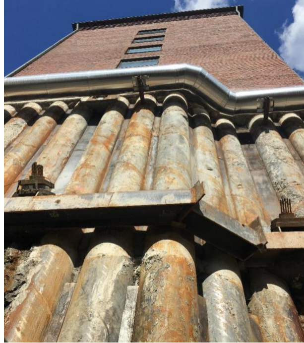
Figure 15: Pipe piles installed using Spiral Flush pilot bit adjacent to the 1962 old building
