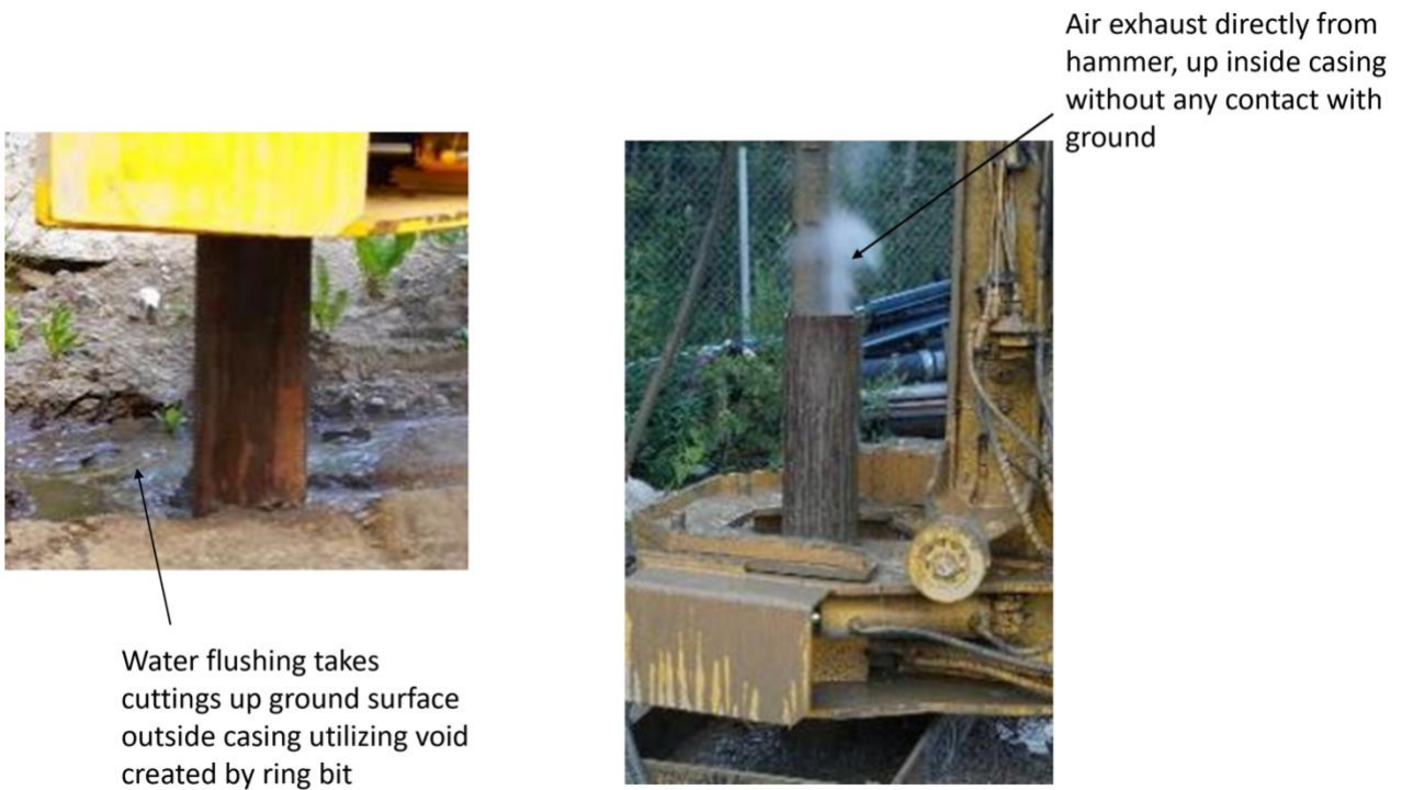
Figure 12: Flow paths of air and water during drilling using the ALF system
