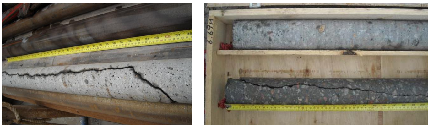
Figure 1: Examples of subvertical crack observed on concrete cores of bored piles
