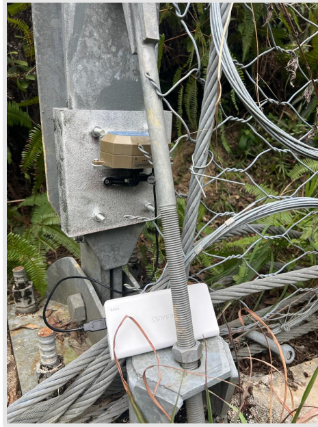
Plate 3: Photo of Sensor Charging using power bank
