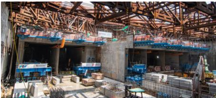
Figure 19: Anti Drag System with strand jacking restraint
