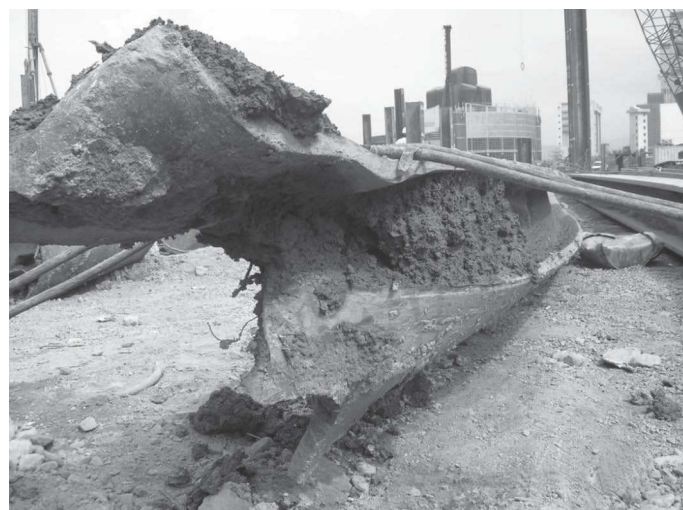
Figure 6 – Photo of Some Damaged Piles
