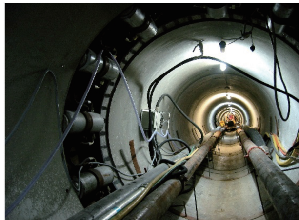
Figure 8. Appearance of a jacked tunnel with intermediate jacking station and automatic lubrication system.
