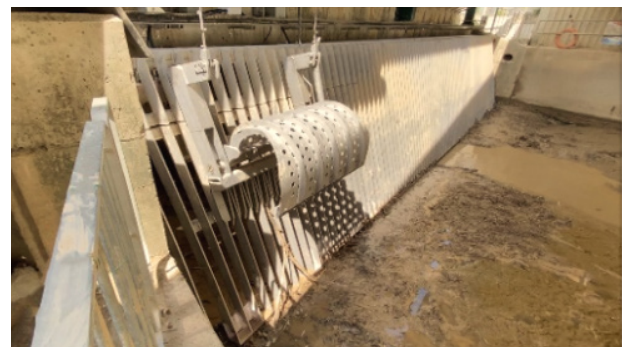
Figure 4. Mechanical grab system at the Kong Yiu Channel.
