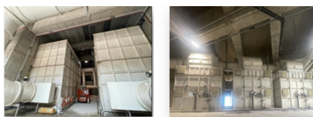
Figure 7. Bio-trickling tanks (left) and activated carbon filters (right).
