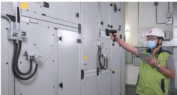
Figure 4. RFID tag installed at an E&M asset.
