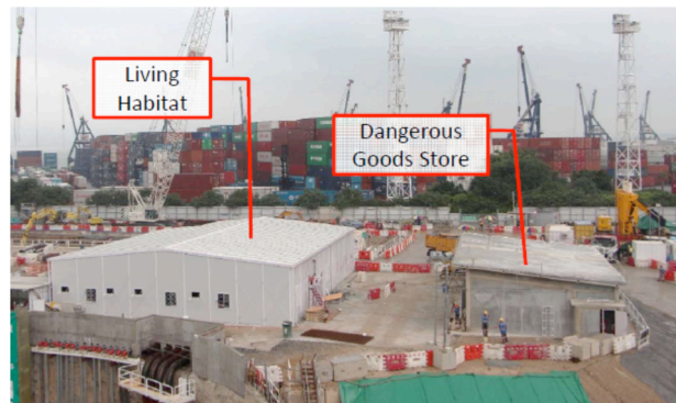
Figure 4. General view of Living Habitat and Dangerous Goods Store for trimix gas.
