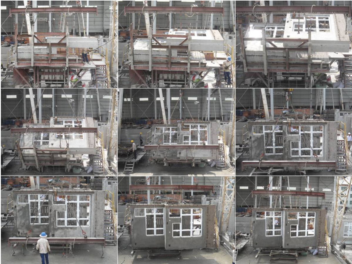
Figure 3.17 Sequence of lifting of a precast façade (from top and left to right).
