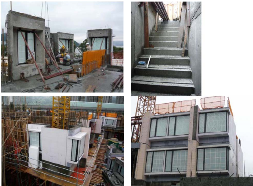
Figure E.13. Precast Elements
