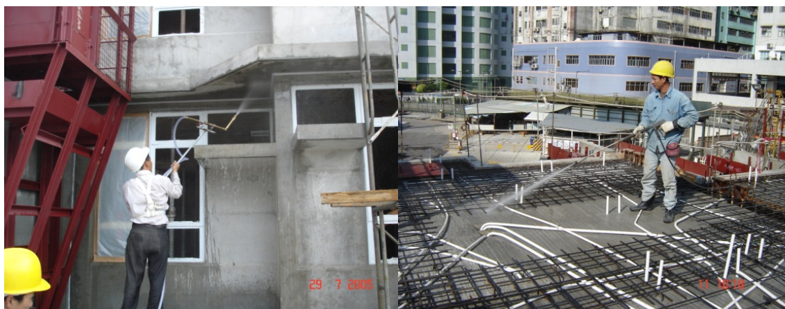
Figure A1 Watertightness test on the mock up on the precast units.
