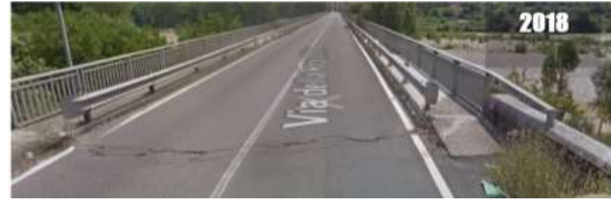
Expansion cracking of asphalt concrete pavement on a bridge
