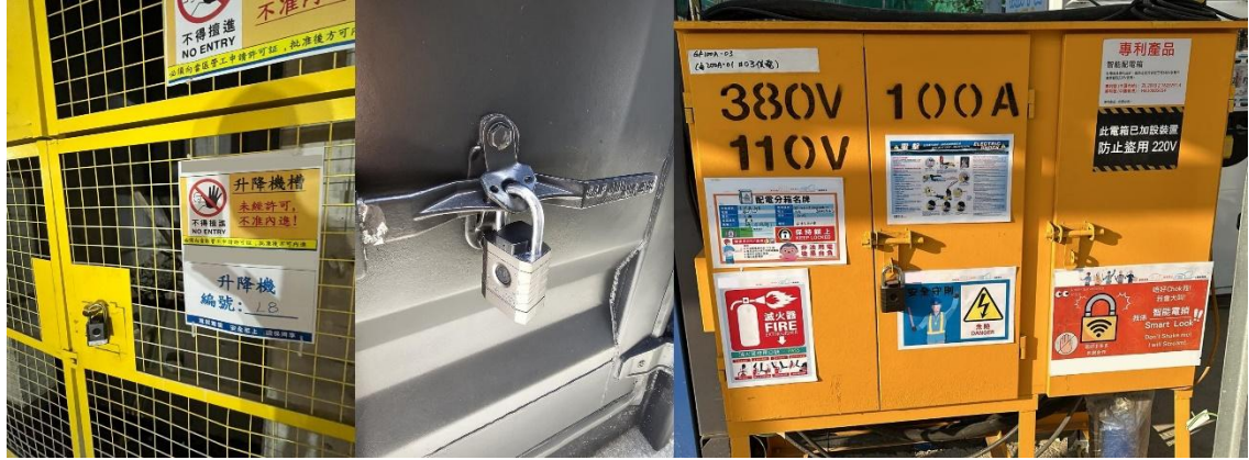
Figures 6, 7 & 8 – Example of E-lock Authentication on Lift-Shaft (Left), Storage Room for Dangerous Goods (Middle), and Electrical Box (Right)
