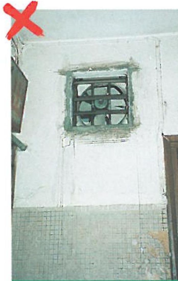
Unauthorized opening in fire resisting wall and the installation of exhaust fan
