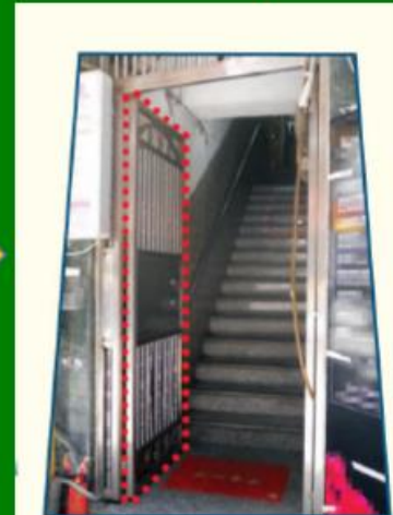
Metal gate obstructing the means of escape
