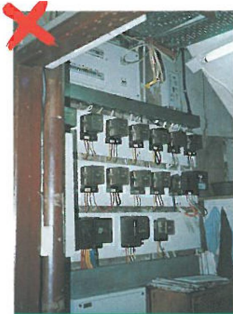
Unprotected electric meter room
