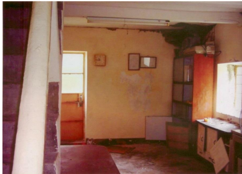
Sacristy before renovation was full of defects
