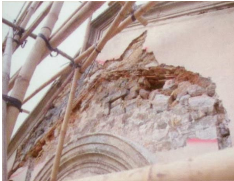
Defects found at the external wall of the front façade of the Chapel
