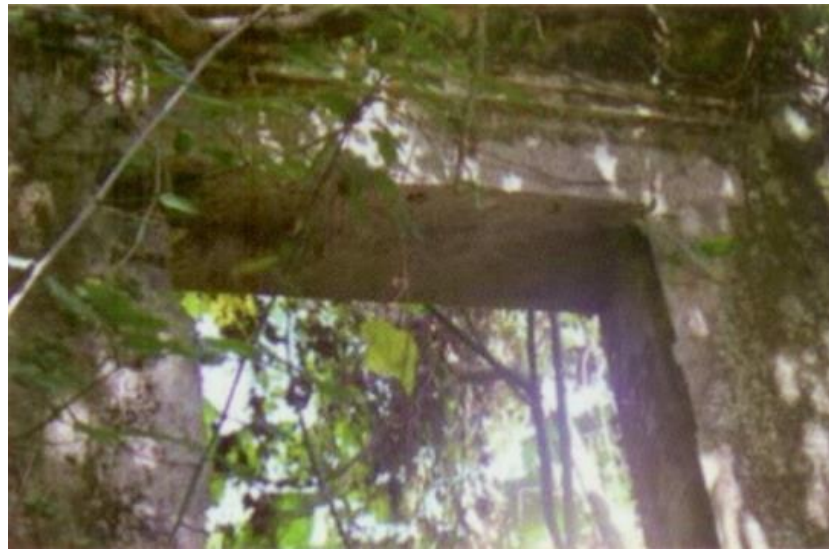
Close-up of the window frame of the rear wall of the ruined chapel
