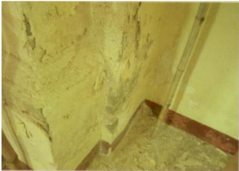
Wearing off of plastering
