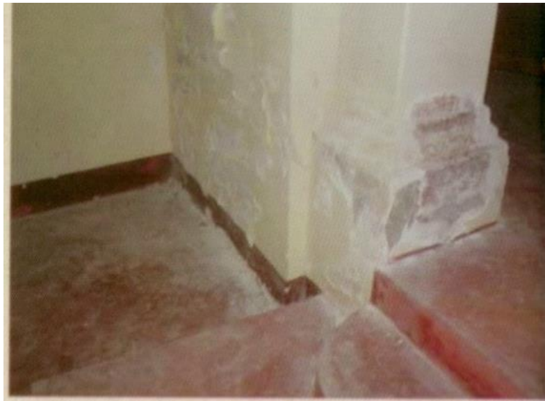
Exposure of the structure as the protective finishing worn off
