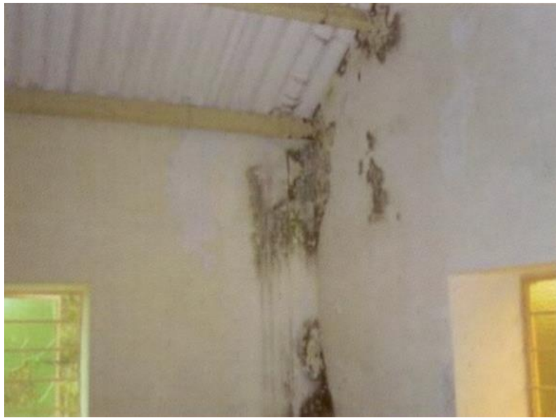
Mold found at the damp corner of the roof
