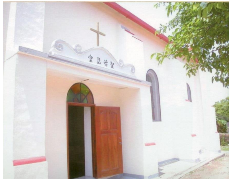
Side door at South-Eastern elevation replaced by timber door of period design after renovation
