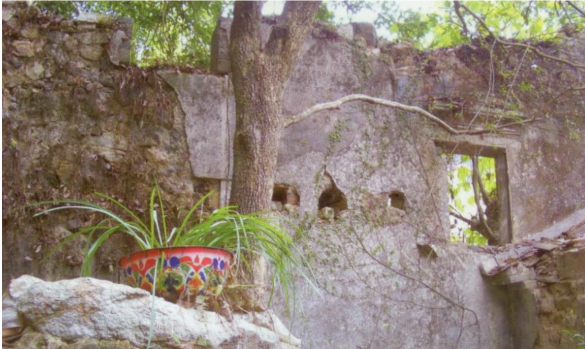
The collapsed wall suspected to be the rear facade of the old St. Joseph's Chapel
