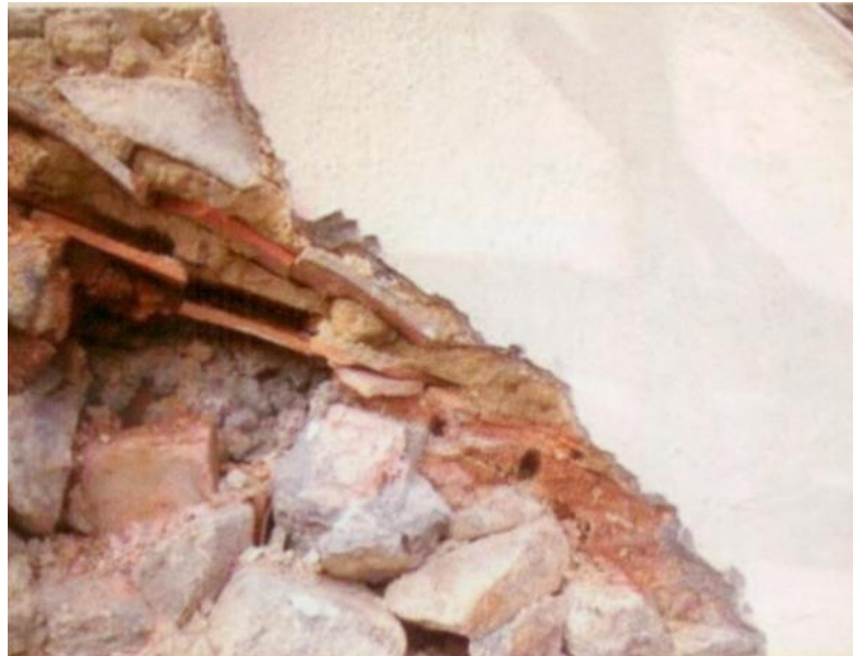
Defects found at the external wall of the front façade of the Chapel
