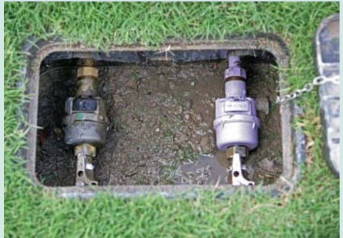
Fig C4.8 Separate meters for potable water and Class A+ recycled water (Purple)
