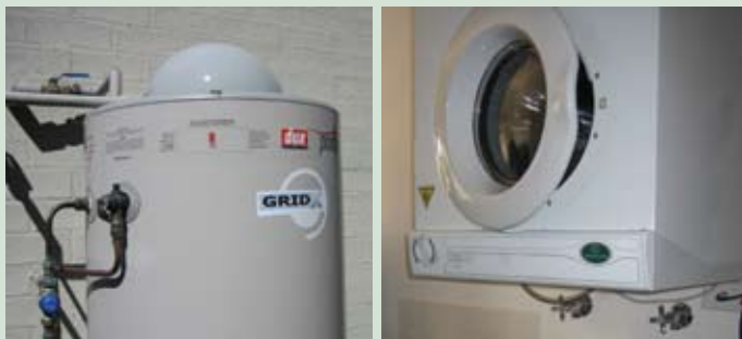
Fig C3.2b Hot water and heat for dry cleaners are generated from the 'Tri-generation' system
