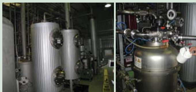
Fig C3.12 The process units
