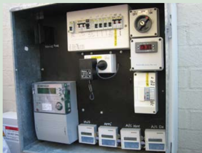
Fig C3.3 Meter cabinet fitted with smart meters recording customer's energy consumption
