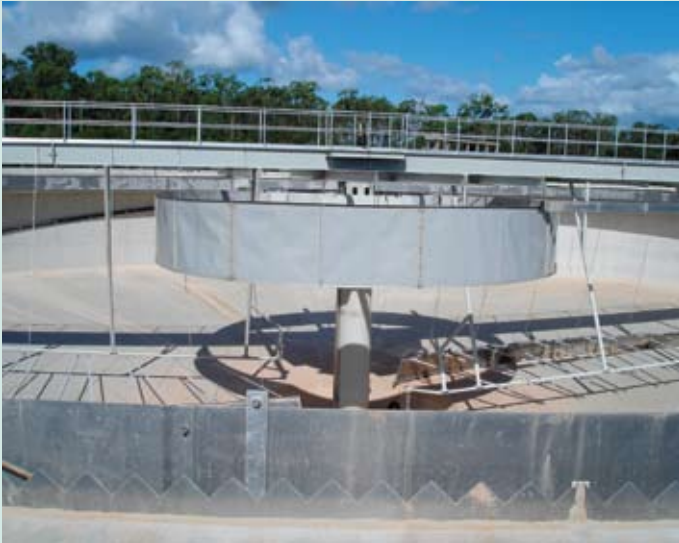
Fig C4.13 Sedimentation tank of the wastewater treatment plant
