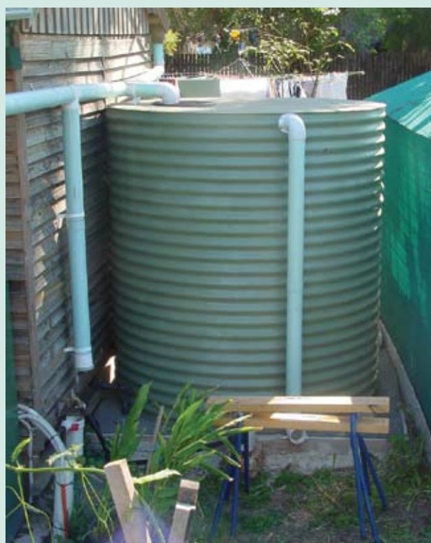
Fig C4.17 A traditional rainwater tank
