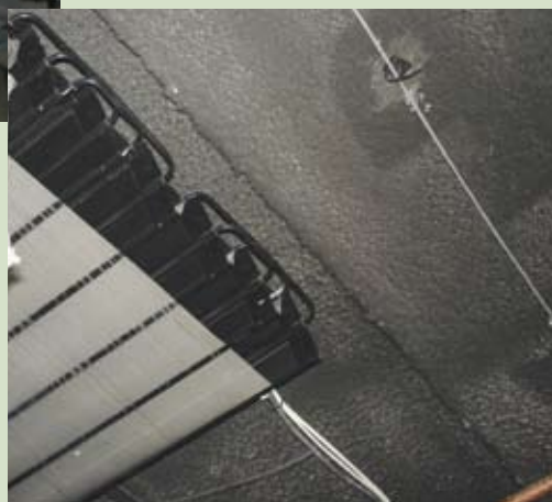
Fig C2.14 Cooling coils and fins of Passive Chilled Beam inside ceiling void
