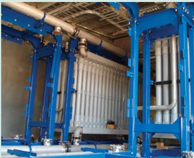
Fig C4.14 Ultra-filtration units of the wastewater treatment plant
