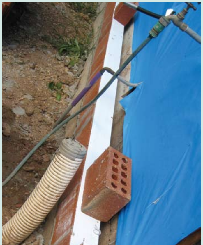
Fig C4.9 Purple pipe for Class A+ recycled water leading into the house
