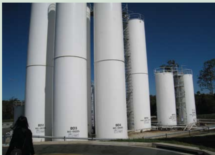
Fig C3.11 Feedstocks and final product storage tanks
