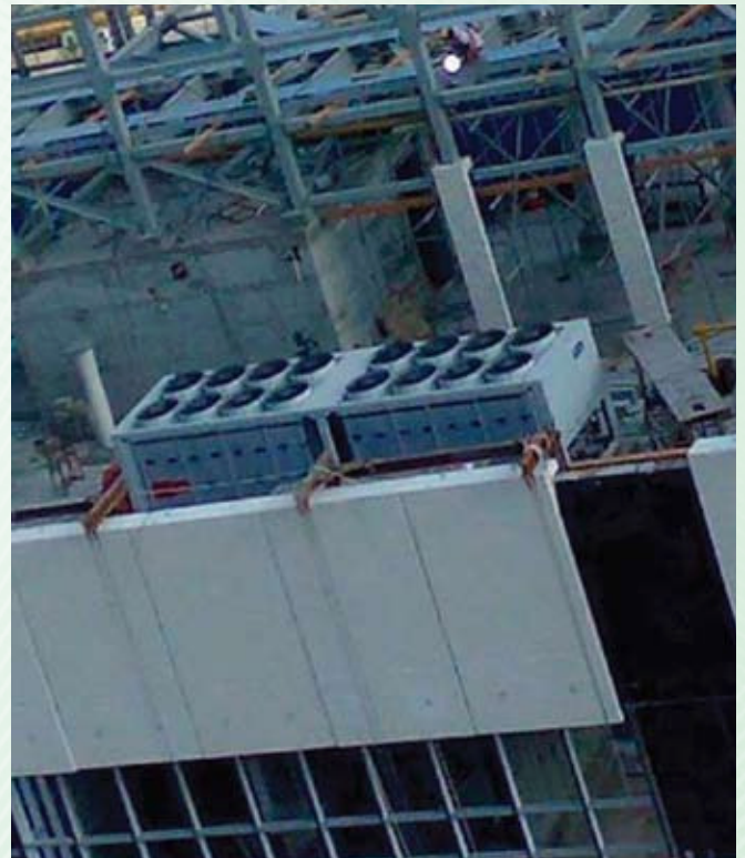
Figure 4.1.2 Chillers in building [1]
