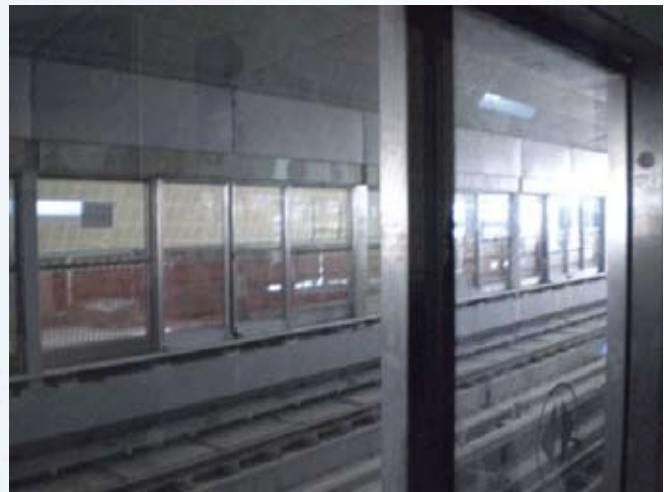
Figure 3.3.19 Platform screen doors
